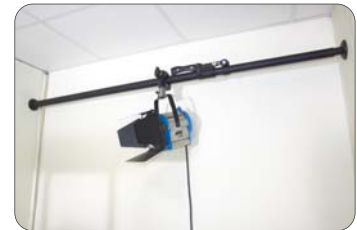
Horizontal for lighting
